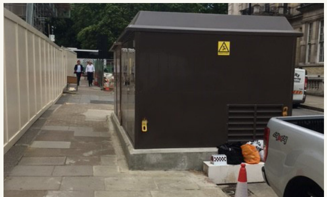
View of Temporary Substations July 2017
